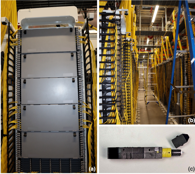
Figure 8: (a) One of the racks hosting the emulated ShuffleBoxes. (b) Rows of emulated ShuffleBoxes. (c) A ShuffleBack dongle with 4-FPs MPO connector.
